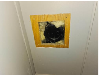
Innvendig stakeluke - Stakeluke
