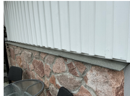
Noe bom/hullyd under skifer
