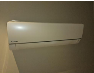
Varmepumper - Plassert i trapp.
