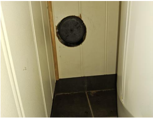
Innvendig stakeluke - Stakeluke
